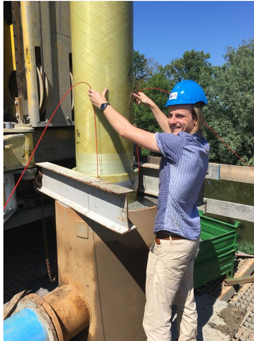
Composite well (GRE) with fibre-optic DTS
