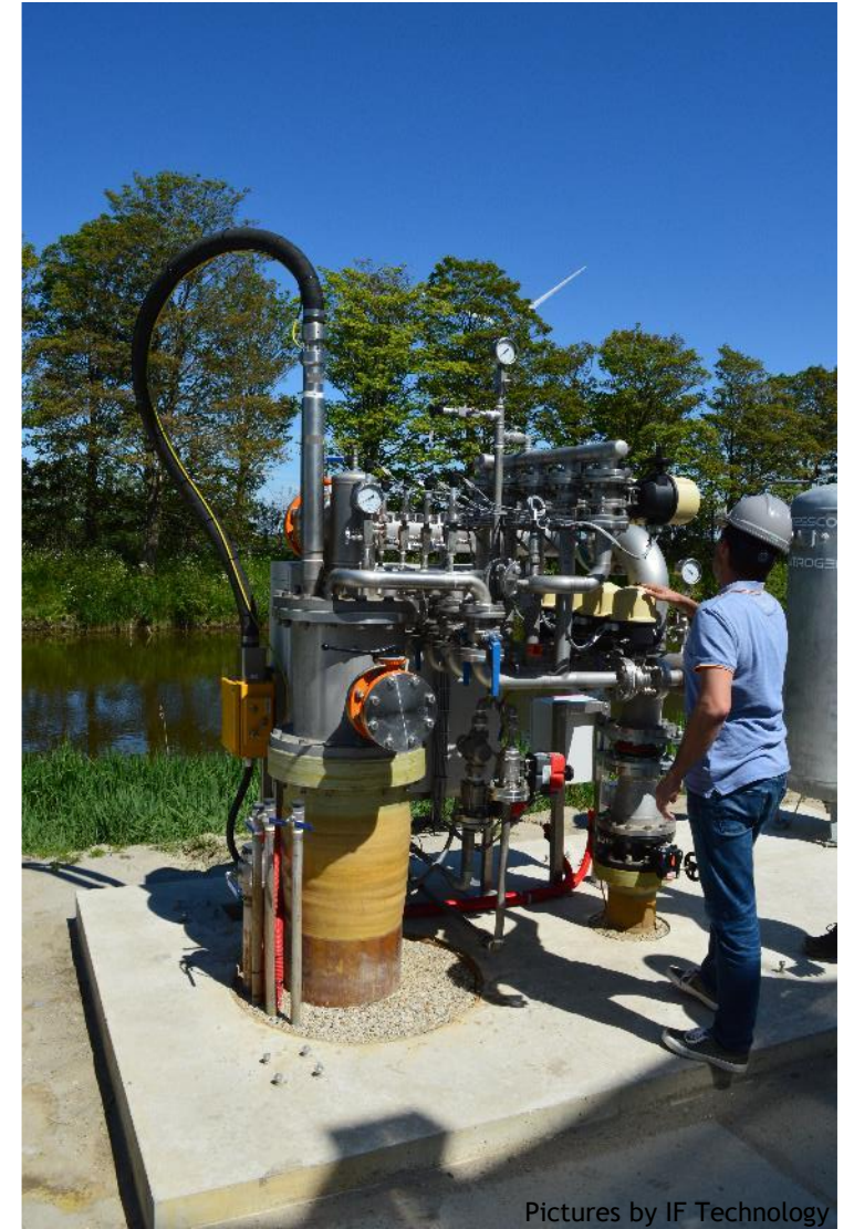
Hot well with piezometers
